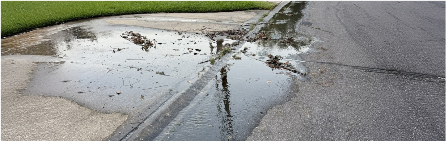
Irrigation audits help prevent irrigation water (and your dollars) from going down the drain. Photo by Eric DeBoer
